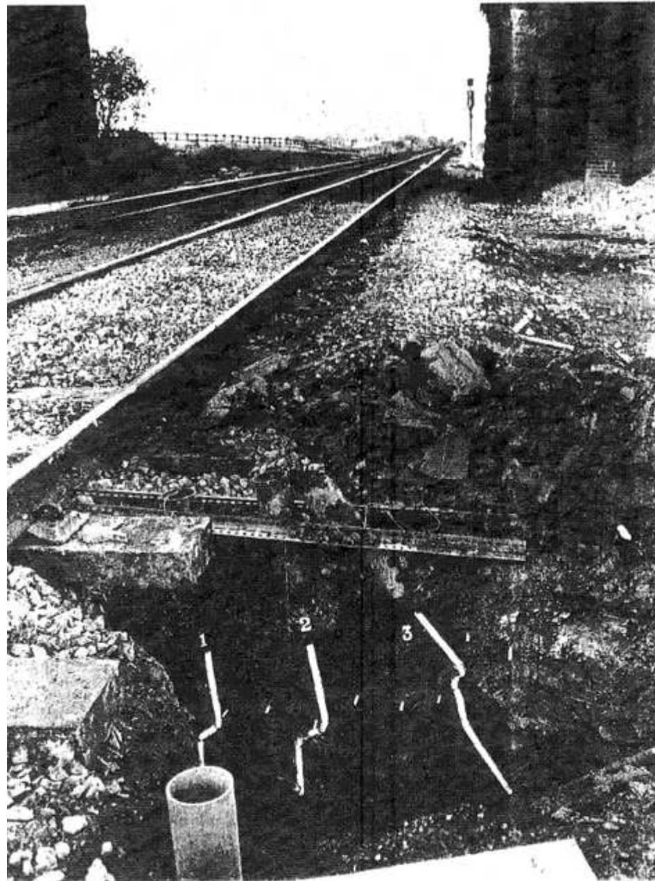
Fig. 6 Distorted columns indicating cess heave failure
